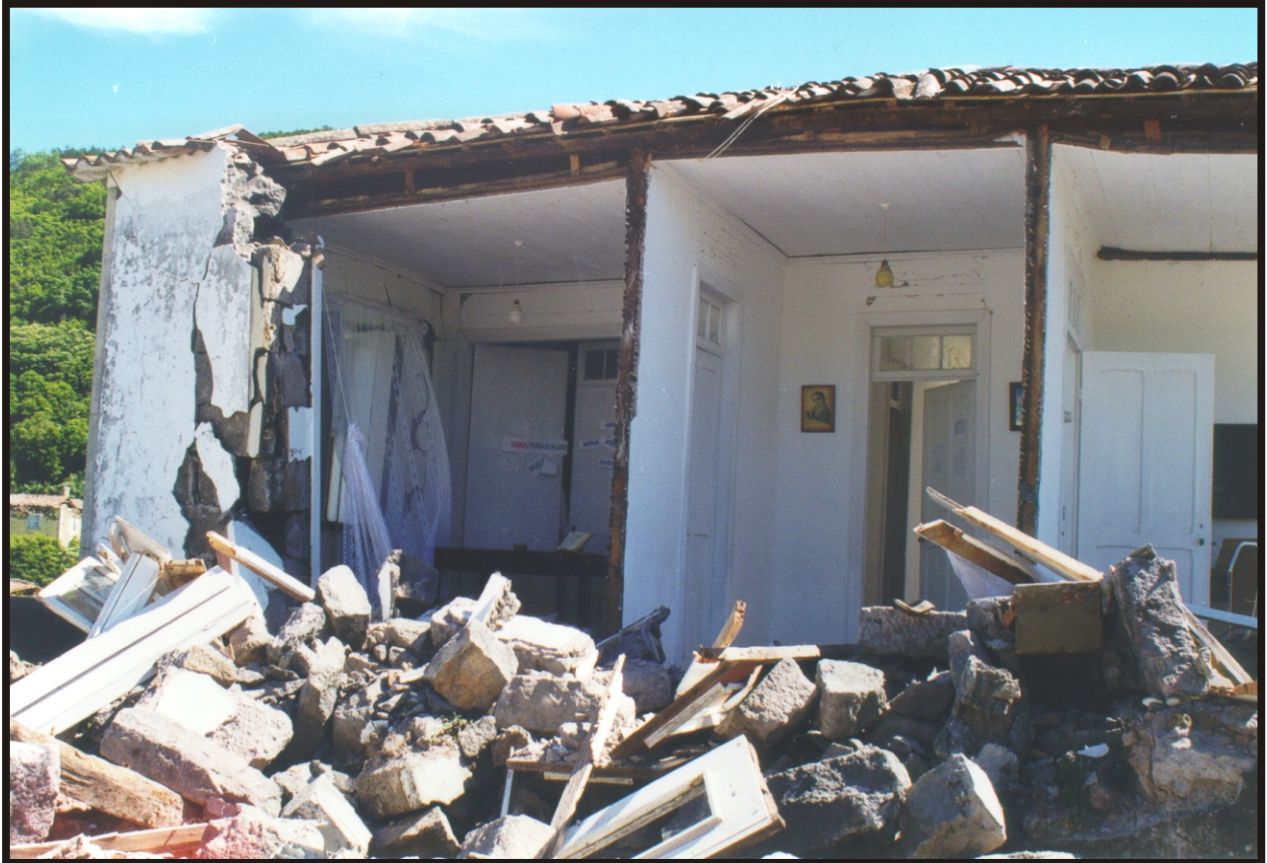
Plate 3. Earthquake damage in the Espalhafatos region from the Azores Islands earthquake 9 July 1998 05:19 UTC, magnitude 6.0 Ms. (Photograph supplied by Mr Fernando Carrilho, Instituto de Meteorologia, Portugal).
