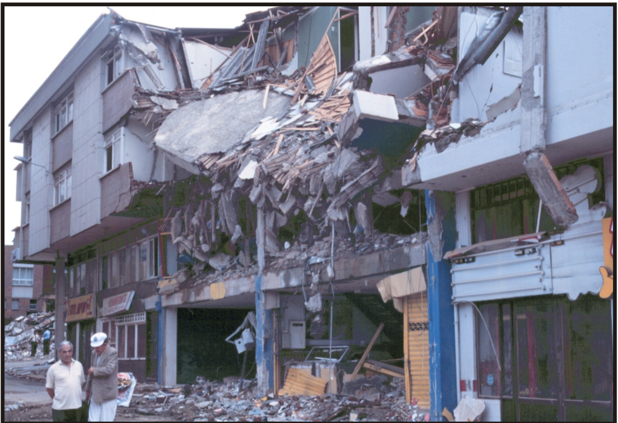
Plate 4. Earthquake damage in the Armenia region from the Colombia earthquake 25 January 1999 18:19 UTC, magnitude 5.9 Mb. (Photograph supplied by Mr Fabio Taucer, European Commission).
